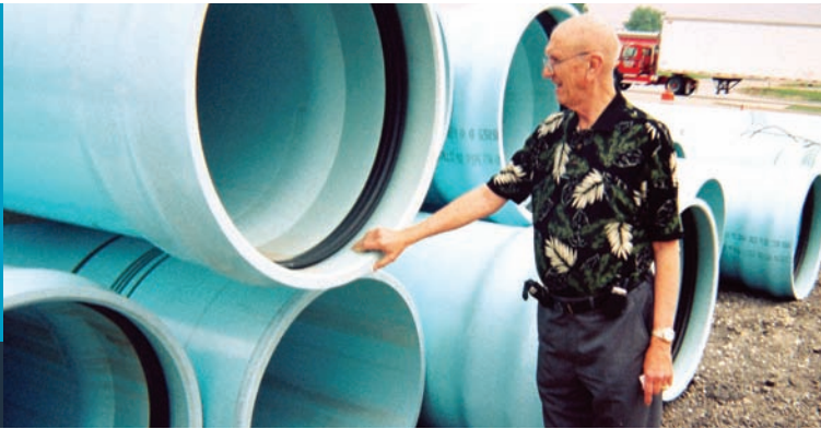
Fred Valenta, with JC Utilities, admires the 36-inch PVC pipe being used to replace the ductile iron pipe.
