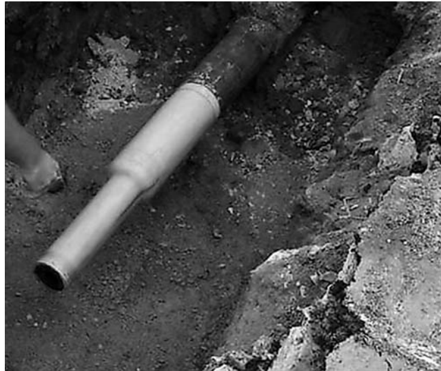
Fig. 13.15 Expanded structural liner with hardware removed.
