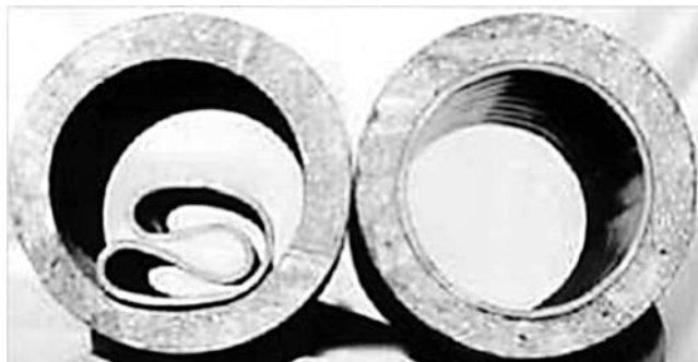
Fig. 13.18 Tight fit PVC liner; inserted is shown on left, expanded is shown on right.
