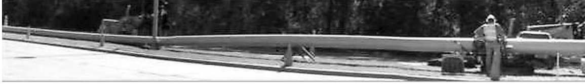
Fig. 13.7 PVC pipe supported on rollers.
